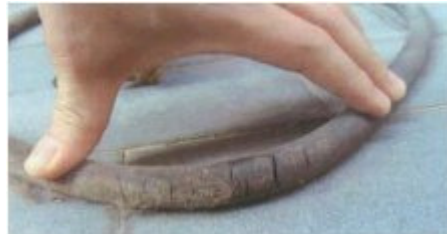
A number of cracks are found on the flexible gas tubing
