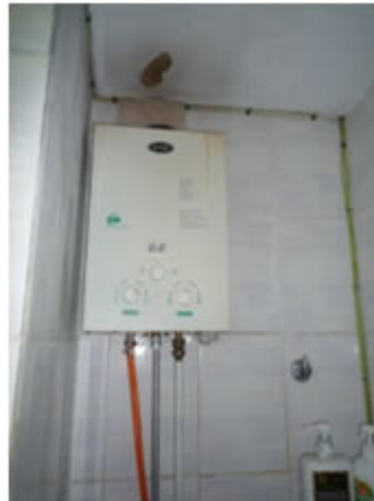
Non-EMSD approved and flueless gas water heater
